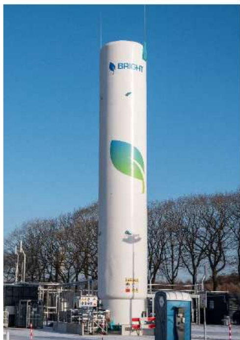
CO 2 -Storage Tank
