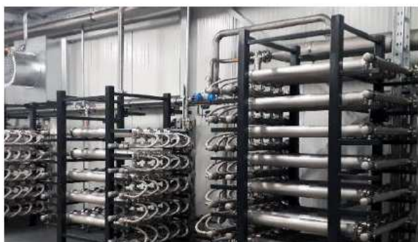
Membrane modules in a building
