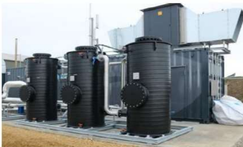
Biogas Filtration System (HDPE)
